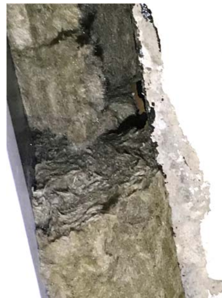
Wetting of installed rockwool
