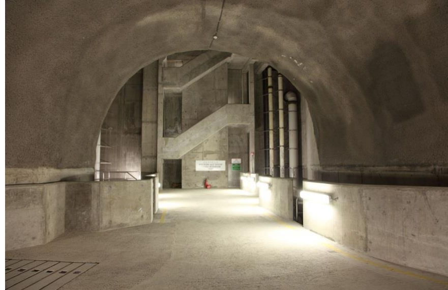
Inside the WSD Western Salt Water Service Reservoir at HKU
