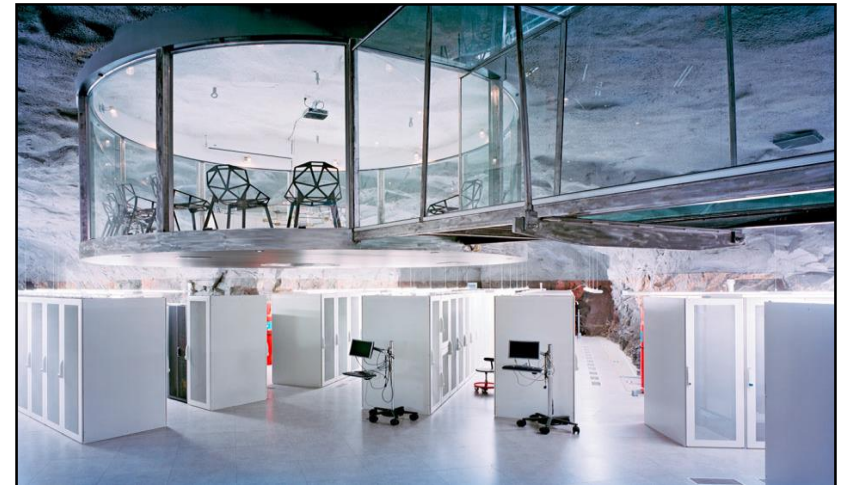
Pionen White Mountain Data Centre with Glass Walkway and Boardroom, Sweden
